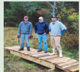
Employees from the Knickerbocker Group keep hikers' feet dry by constructing small bridges at Zak preserve.
